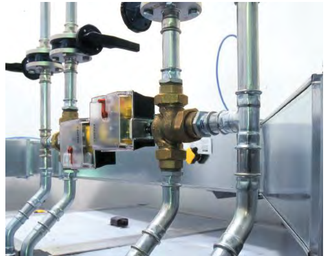
Figure 22 - steelPRES - refrigeration (closed circuit)
